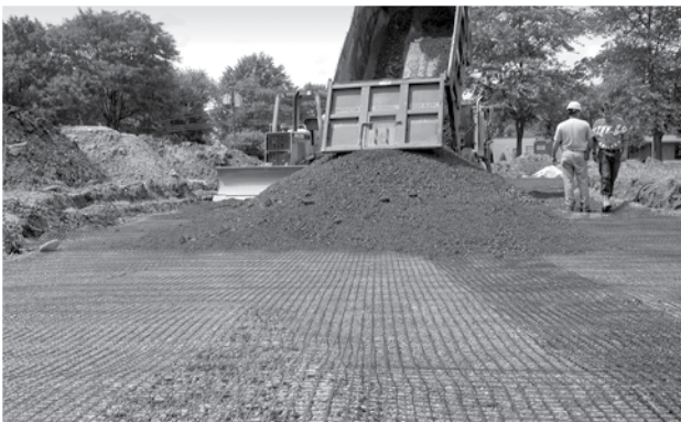
IMAGE 9A: End dumping aggregate fill on top of Tensor Geogrid over soft subgrade.
