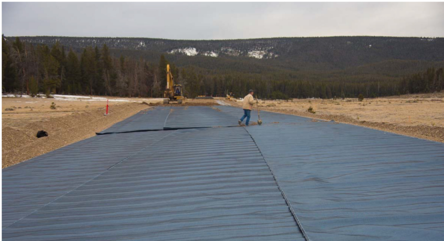
Figure 6: Installation of Mirafi® H 2 Rx with the geotextile unrolled in the direction of the road alignment and the overlapping of geotextile rolls from right to left in a road section with super-elevation on right.
