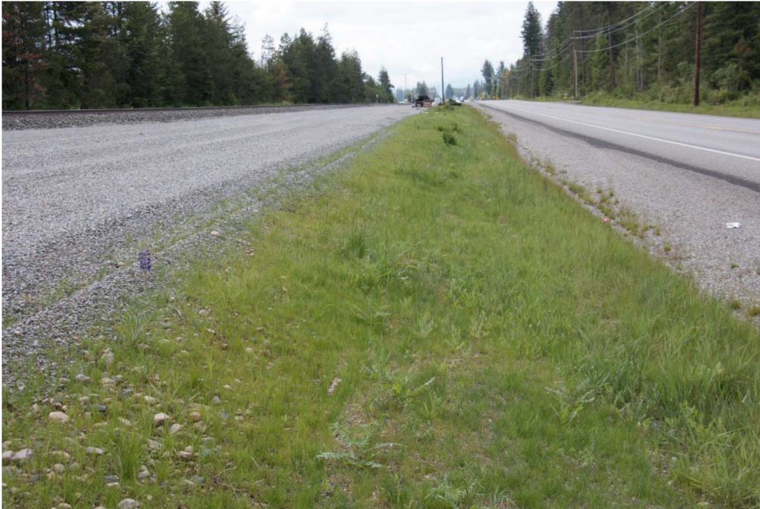
Figure 10(b): Photo of a Mirafi® H 2 Rx road project with draped geotextile tongue beneath a bio-wicking vegetated soil cover.
