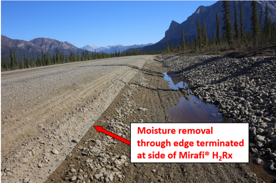
Figure 8(c): Photo of a Mirafi® H 2 Rx road project with geotextile edge terminated at side.
