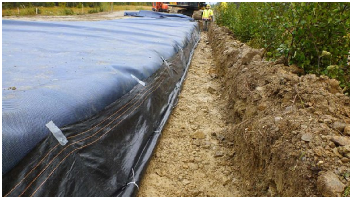
Figure 11(c): Photo of a Mirafi® H 2 Rx road project with geotextile edge terminated in a saw-cut pipe.
