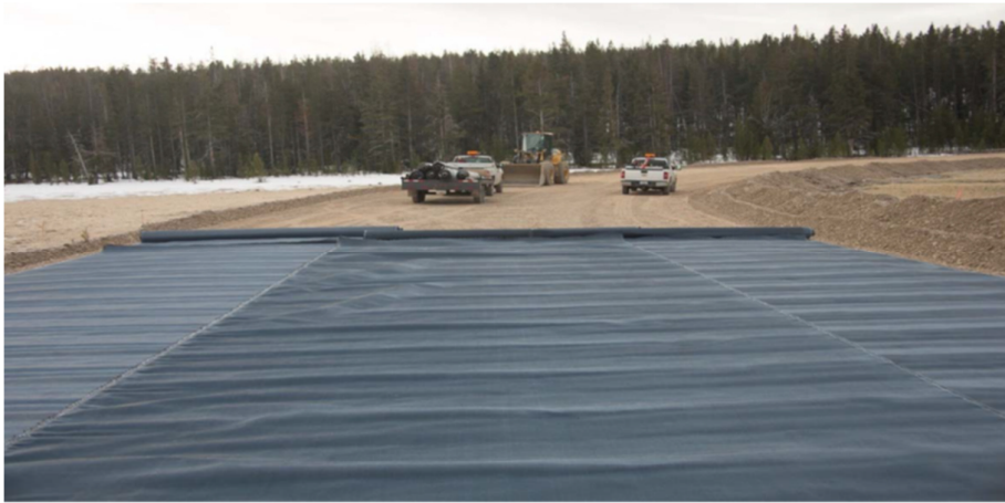
Figure 5. Installation of Mirafi® H 2 Rx with the geotextile unrolled in the direction of the road alignment and middle roll overlapping the two adjacent side rolls in a double cross elevation fall.
